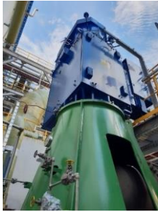
Gambar 6. Hot Well Pump (PGE, 2019)
