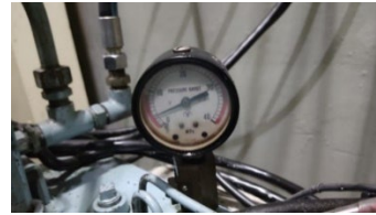
Gambar 8. Pressure Gauge Pompa Moving Bolster
